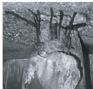
图8 Loma Prieta地震中桩-面板连接破坏 Fig. 8 Damage at a pile-deck connection during Loma Prieta earthquake
